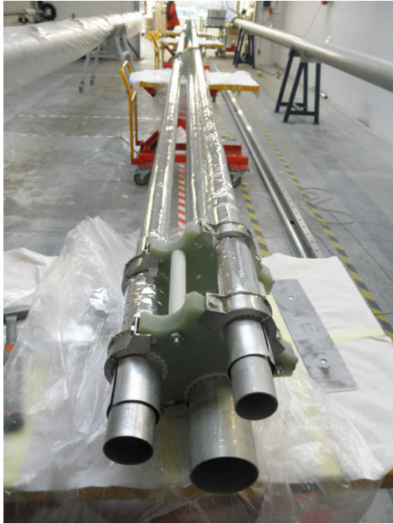
Fig. 9.22 Sliding supports on the XATL1 straight module process lines (courtesy Kriosystem Ltd.)
