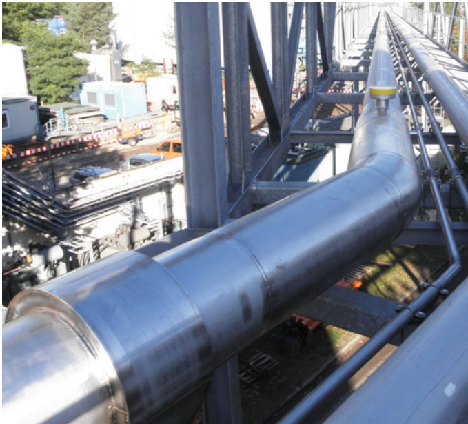
Fig. 9.29 The XFEL/AMTF cryogenic transfer line installed on the pipe bridge ( courtesy Kriosystem Ltd.)
