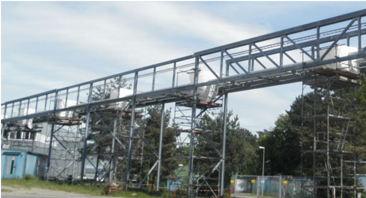
Fig. 9.27 The XFEL/AMTF cryoline interconnections on the pipeline bridge protected with tents (courtesy Kriosystem Ltd.)
