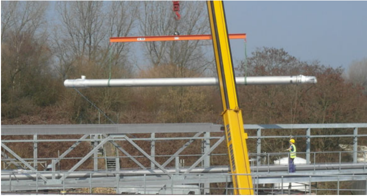
Fig. 9.26 Installation of one of the XFEL/AMTF cryoline straight modules on the pipeline bridge (courtesy Kriosystem Ltd.)
